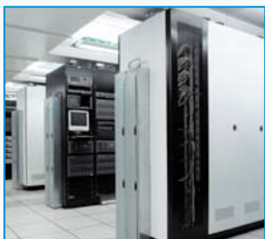
Data centre cooling
