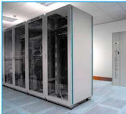
Data center cooling
