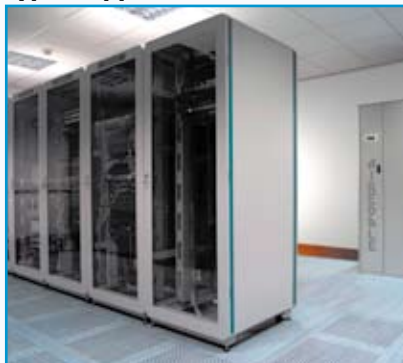
Data center cooling
